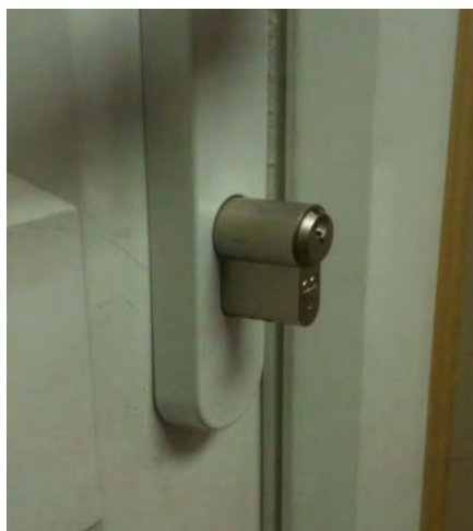
Example of a badly fitted cylinder
